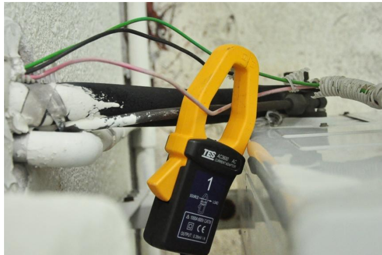
Figure 3.23: Current measurement using current transducer
