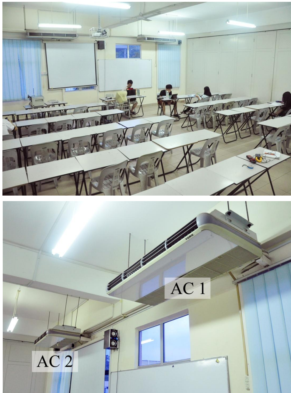
Figure 3.12: AC 1 and AC 2 inside the classroom
