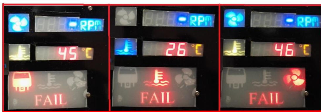
Figure 4.17: Failure indication (From left to right – Relay Fail, CTS Fail, Fan Fail)
