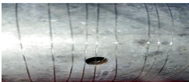
Figure 3.9: Hole on the pipe and cover by a fibre sensor ring to detect the water flow out from the leakage
