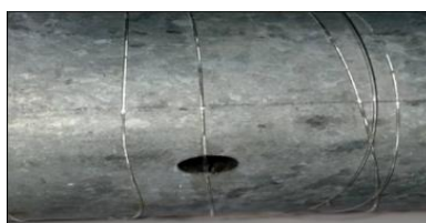
Figure 4.21: Single fibre ring on hole defect
