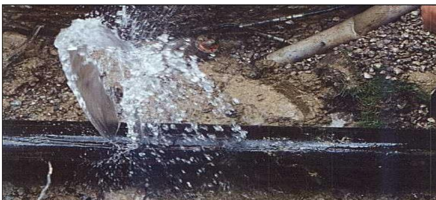
Figure 2.11: Pipeline leakage in daily life ( Water system services , 2016)
