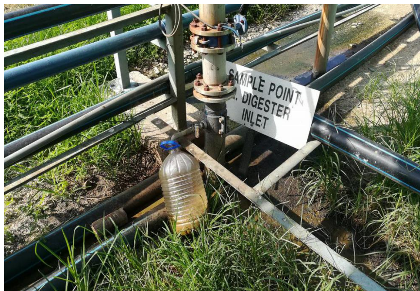
Figure C2: Palm Oil Mill Effluent (POME)
