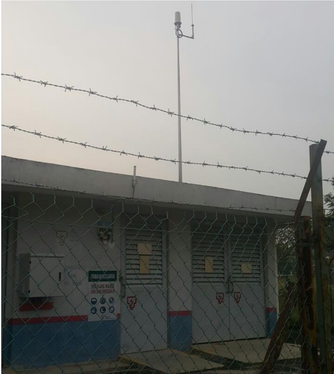
Smart Substation with RF communication tower in the background.
