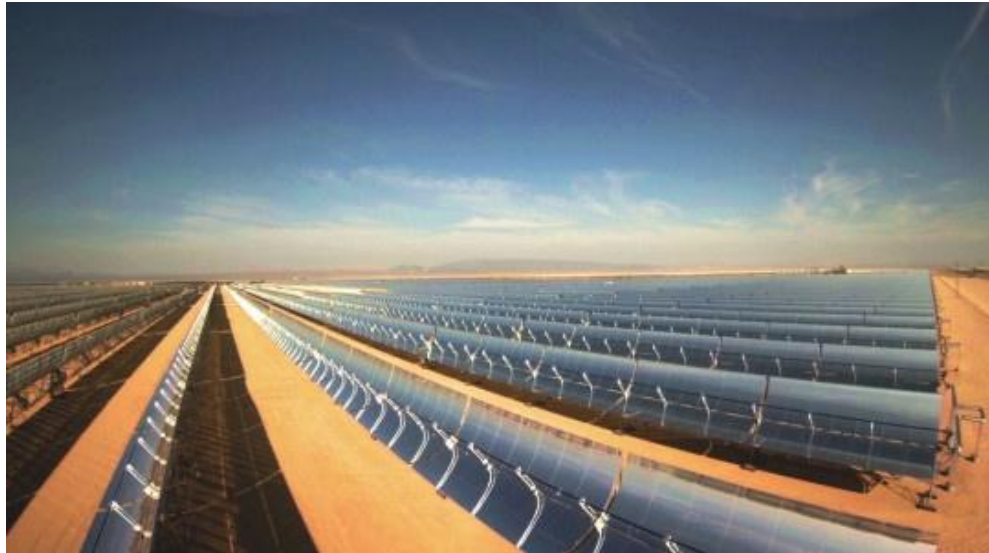
Figure 2.8 Parabolic Trough in MOJAVE
