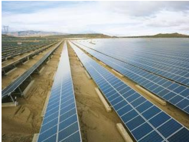
Figure 2.4 Arnedo Solar Plant in Spain (Lewis, 2016)
