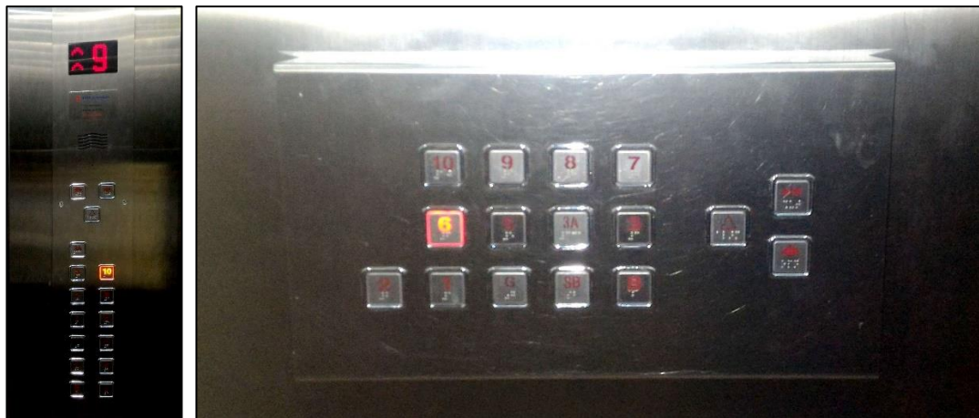
Figure 5.4: Provision of Two Sets of Landing Hall Buttons in the Lift in UTAR KB Block.
