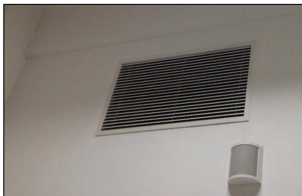
Figure 5.12: Provision of Diffuser or Staircase Pressurization System in UTAR KB Block.
