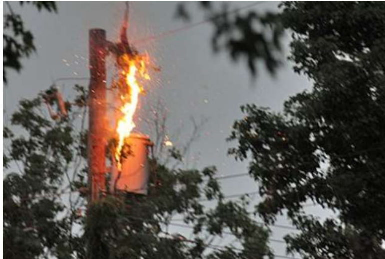
Figure 1-2 An Ameren CIPS transformer is shown exploding caused by lightning
