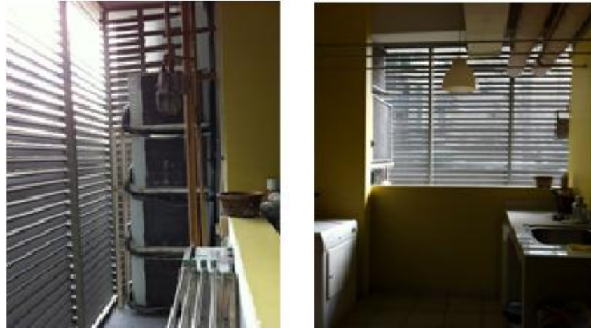
Figure 4.33: Drying area with services location and screened aluminum panels. Image from own source.
