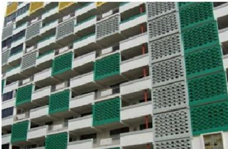
Figure 6.17: Perforated venting hole installed along common corridors. Image from own source.
