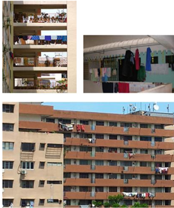
Figure 6.12: Exposed laundries along corridors. Common sights in public low cost housing. Image taken from own source.
