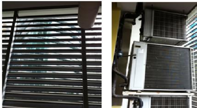
Figure 4.32: Condensers location at balcony of the drying are been screen off by aluminum grills panel. Image from own source.
