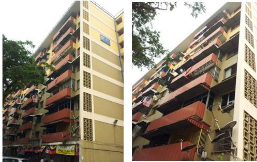
Figure 4.37: View of “Add on” aluminum screen panels screening off the existing open balcony. Image from own source.
