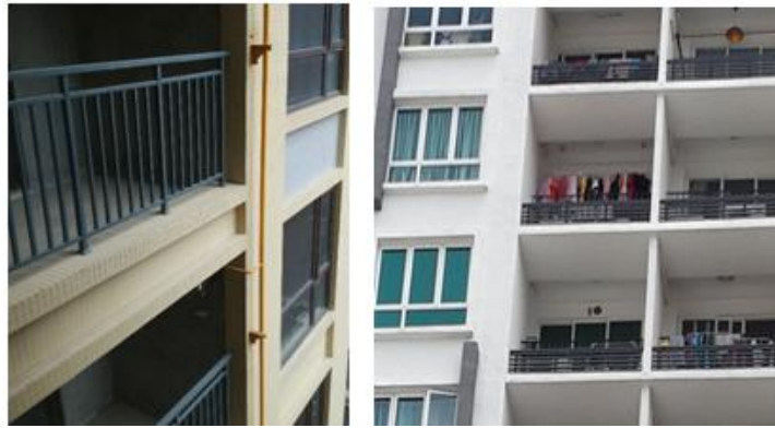
Figure 6.1: Existing exposed balcony with iron grilles railings. Image from own source.
