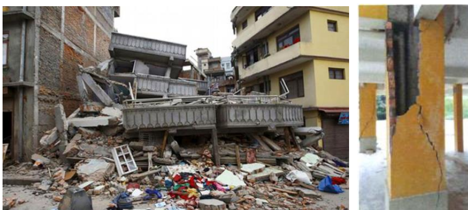
Figure 2.3: Building Collapse (left) (Center For Excellence in Disaster Management & Humanitarian Assistance, 2020) and Cracked Column at SMK Ranau Teacher's Flat (right) (Tongkul, 2016).
