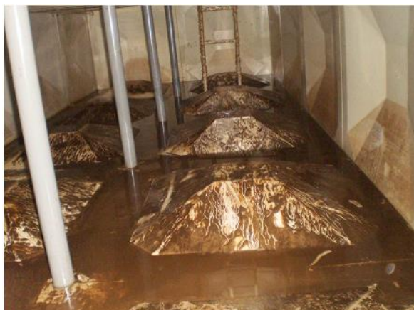
Figure 1.3: Dirty water storage tank due to deposits and sedimentation (Starawaterhygiene, 2020)
