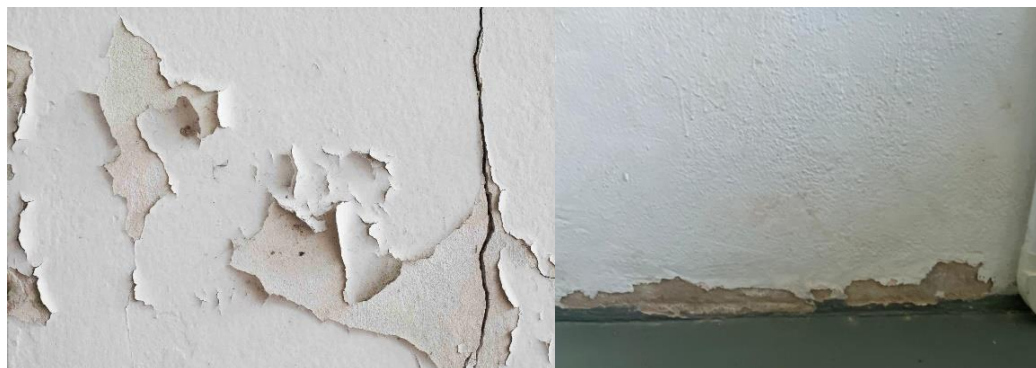
Figure 2.2: Paint Peeled and Faded on Walls
