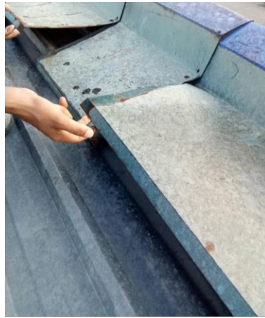
Figure 2.8: Roof Flashing Defect
