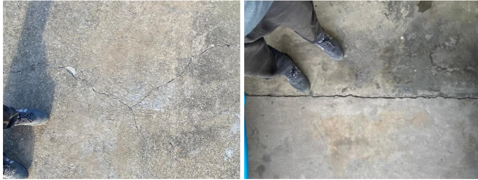
Figure: 2.6: Cracks on Floors
