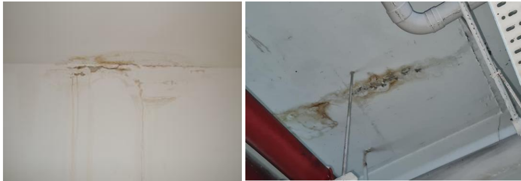
Figure 2.3: Dampness on Ceiling & Slab
