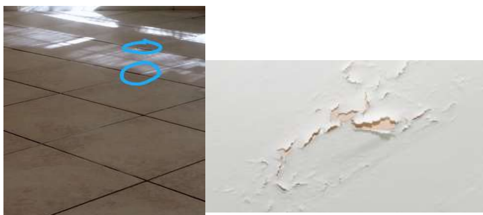
Figure 3. 1 Uneven wall/floor finishing
