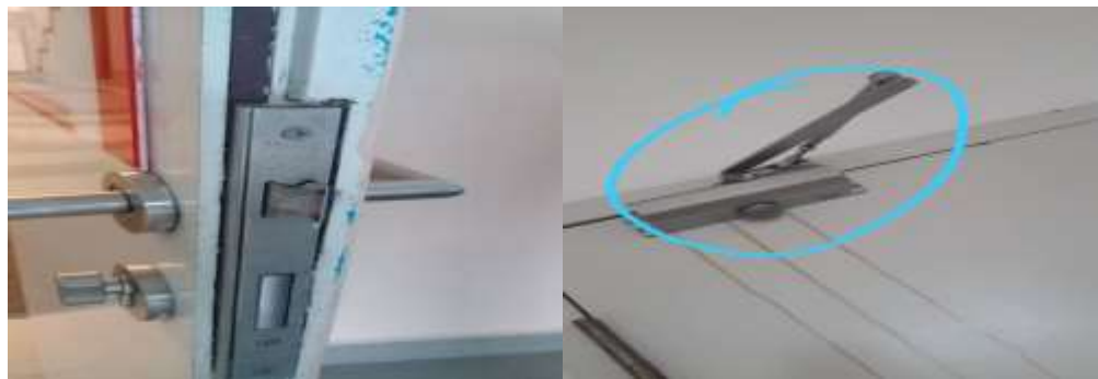
Figure 2. 6: Faulty door handles/door closers
