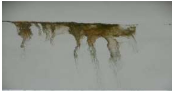
Figure 2. 8 Dampness at the concrete wall
