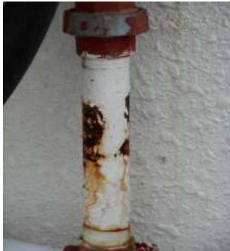
Figure 3. 5 Rusty Galvanised pipe
