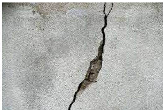
Figure 2. 7 Cracking in building external wall
