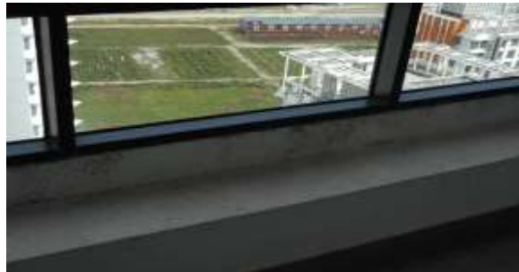
Figure 3. 3 Faulty window gasket
