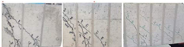
Figure 2.8: Crack Pattern For Specimens With Only FRP Reinforced (Ibrahim, Wakjira and Ebead, 2020)
