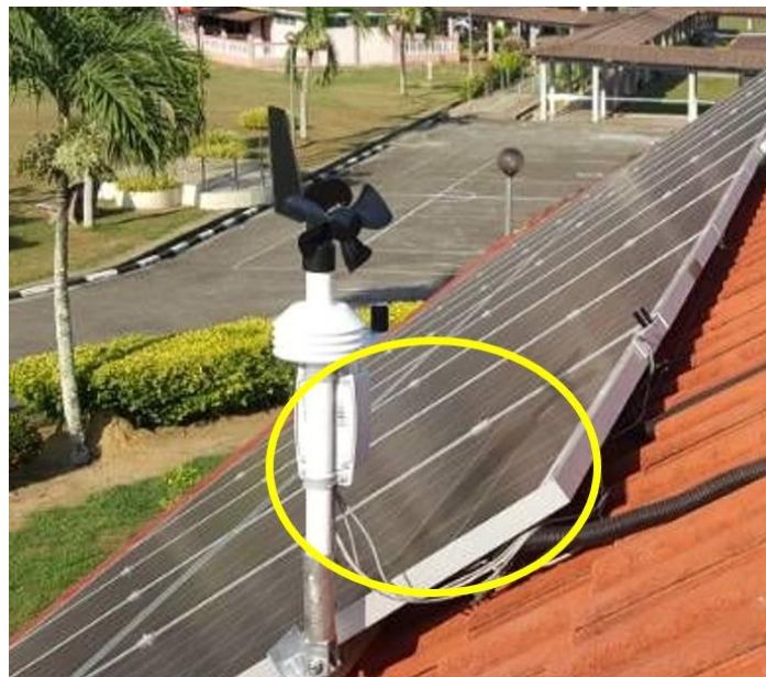
Figure 4.19: An example of wrong installation of weather station.
