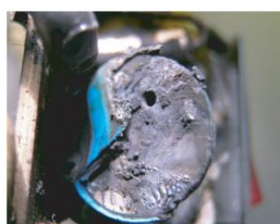
Figure 2.21: Overheat issue blows up the MOV
