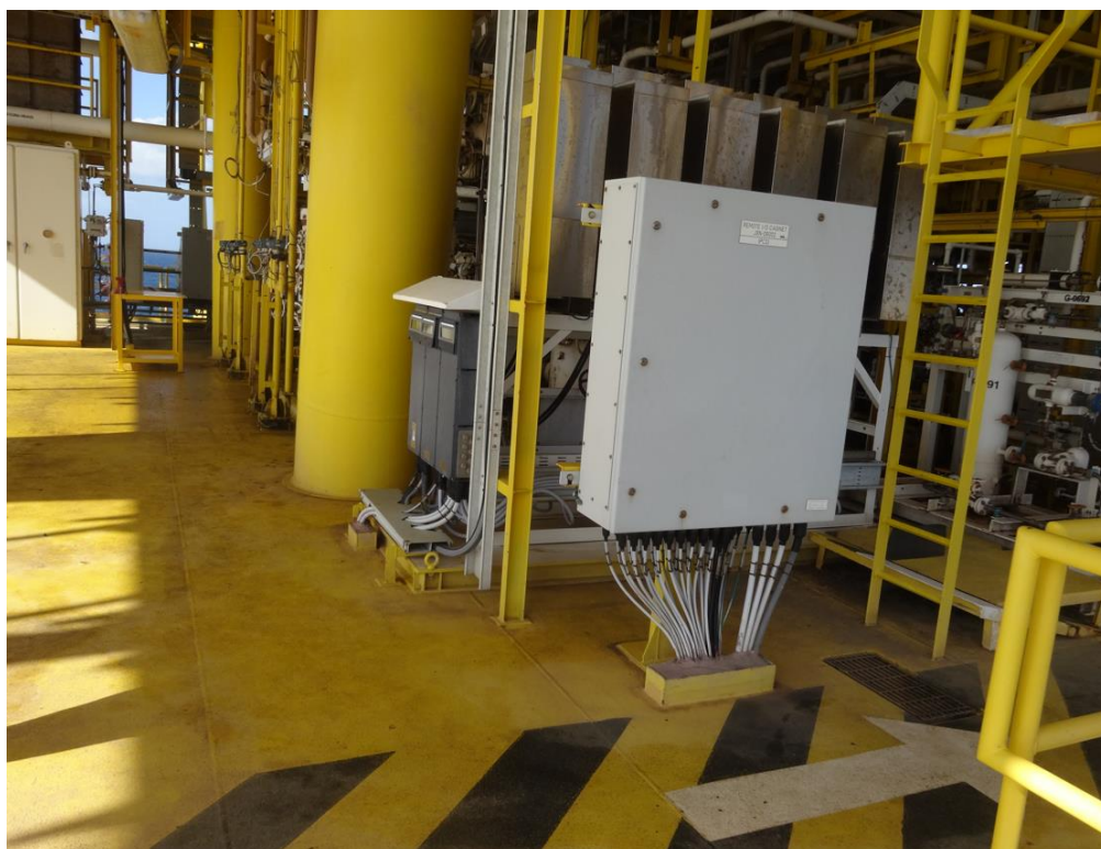
Figure 5.1: Remote DCS IO Cabinet
