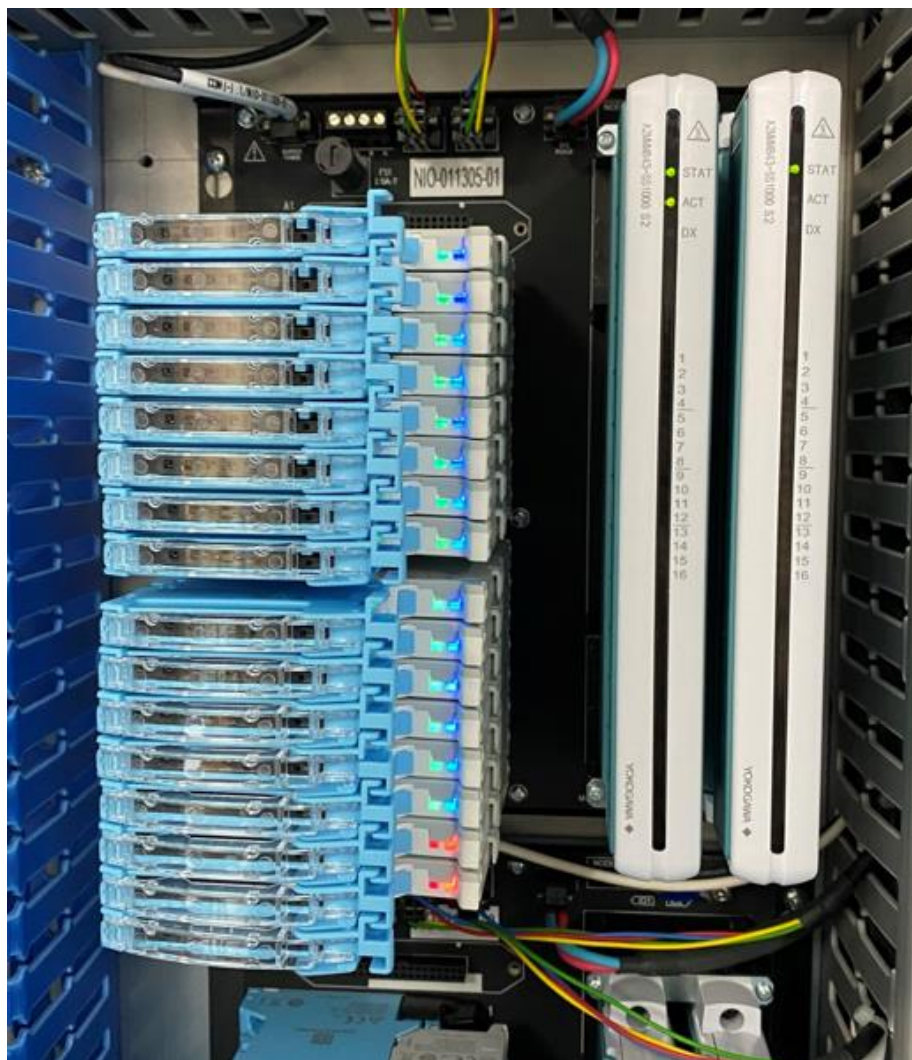
Figure 4.10: Marshalling cabinet configuration with Sum5 and Yokogawa IO card
