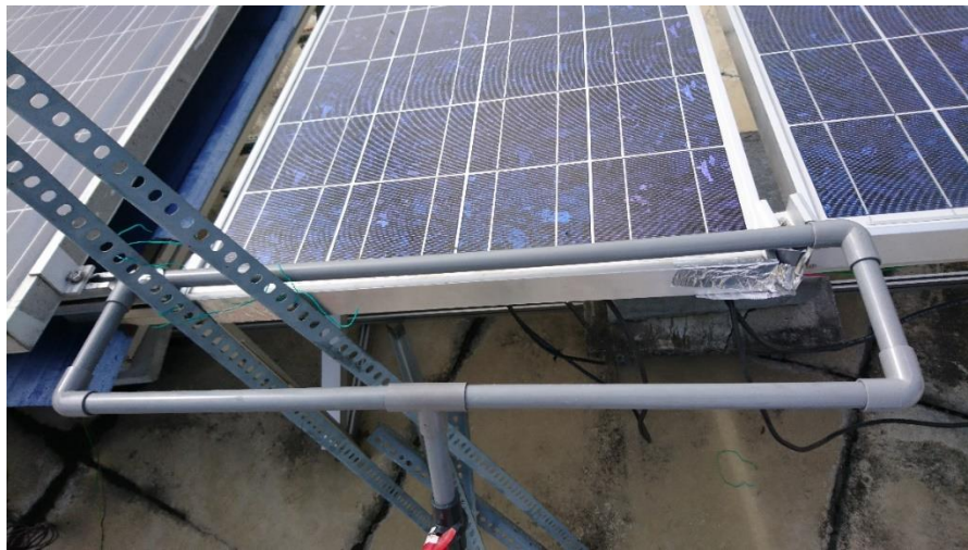
Figure 10: Setup of the water outlet pipe above the PV panel.
