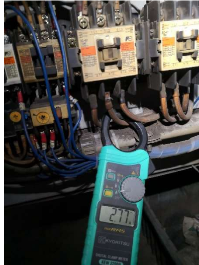
Figure 4.2: Phase current measurement using clamp meter
