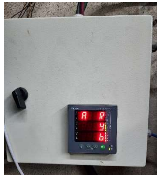
Figure 5.1: Power quality meter panel
