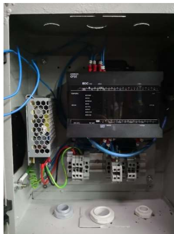
Figure 3.5: Programmable logic controller panel
