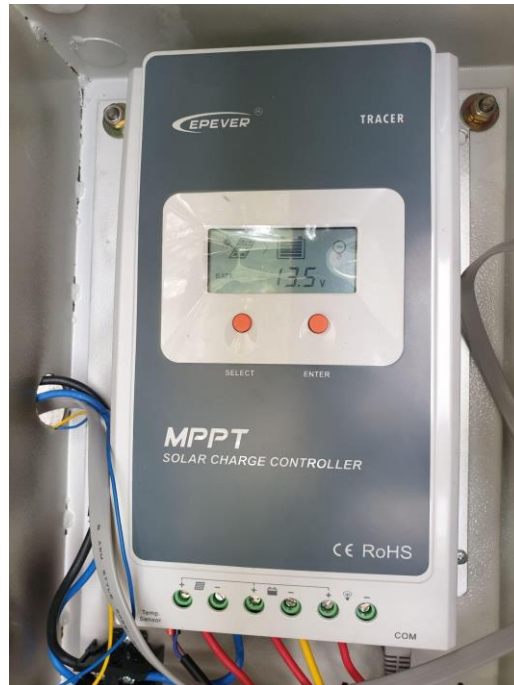
Figure 3.3 Solar Controller - Charge battery and supply constant 12 V
