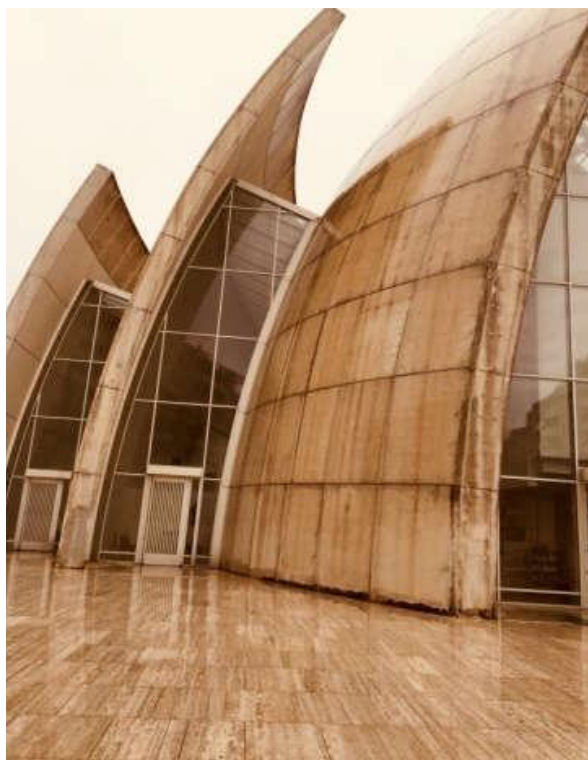
Figure 2.6: External Walls of Church After a Period of Time (Serpone, 2018)
