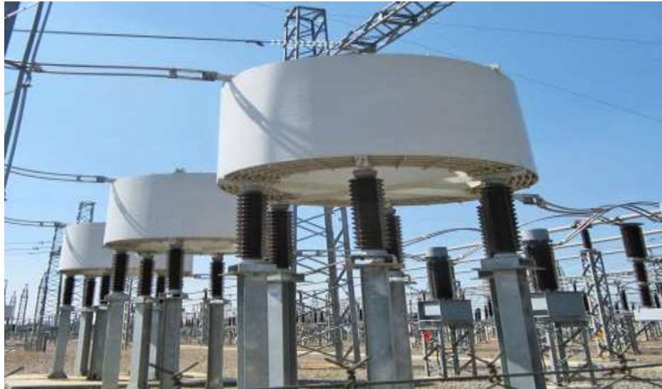
Figure 2.6: HVDC Smoothing Reactors
