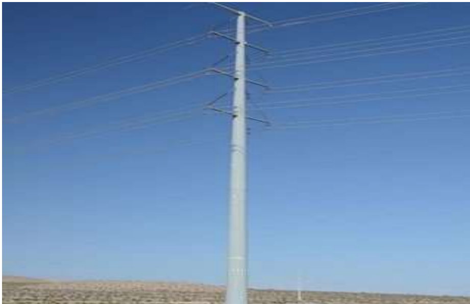
Figure 2.19: Monopolar Power Transmission Tower
