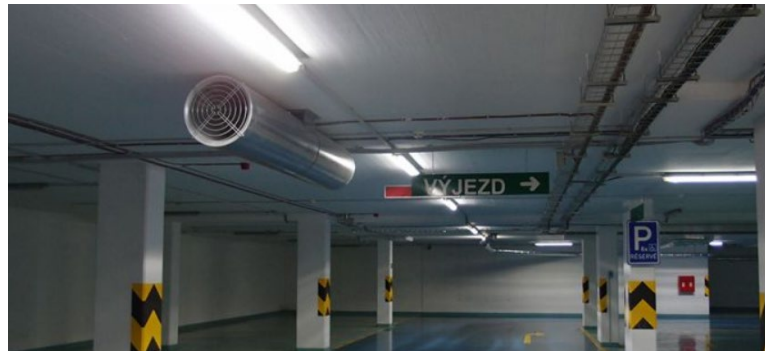
Figure 2.18: Impulse jet fans ventilation system in an underground car park (Colt Singapore, 2022)
