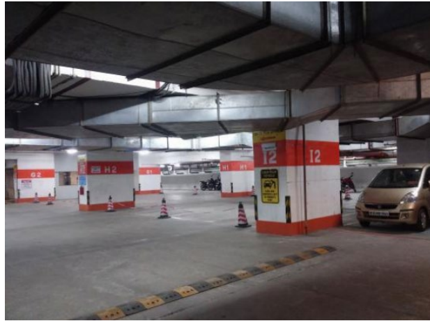
Figure 2.16: Ducted ventilation system in car park (Colt International Ltd, 2020)
