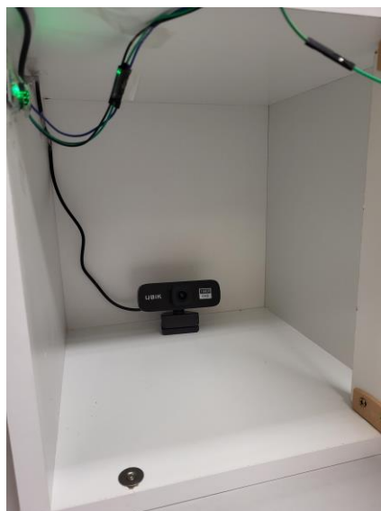
Figure 5.1.1.5 USB webcam placed inside the parcel drop box enclosure
