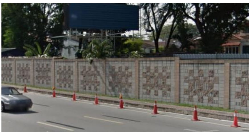
Figure 2.5: Masonry Noise Barriers Employed in Highway Noise Reduction (DOE, 2019).
