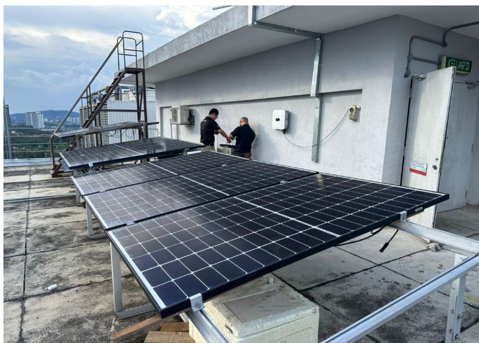
Figure 3.17: PV site on the UTAR Sungai Long Campus KB Block Roof Top
