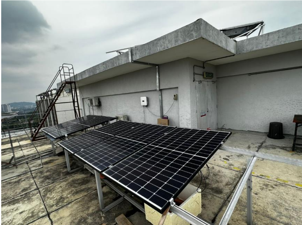
Figure 4.3: PV site setup on UTAR Sungai Long Campus KB Block rooftop for DC arc testing.
