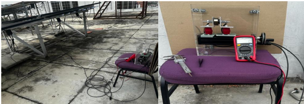
Figure 4.7: Testing setup for DC series arc faults
