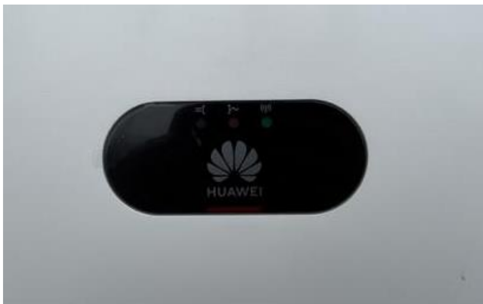
Figure 4.26: Red LED lights up for AC circuit on the inverter
