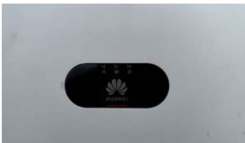
Figure 4.24: Red LED lights up for DC circuit on the inverter
