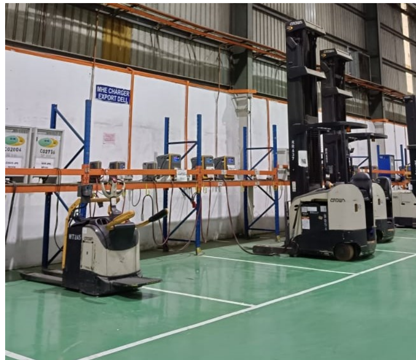
MHE Charging Area.
