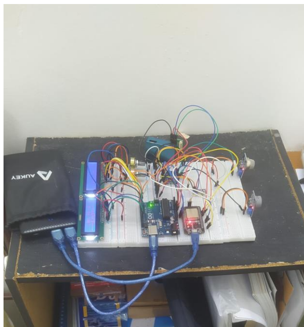
Figure 4.23: The hardware placed at indoor
