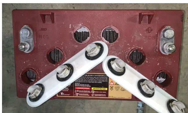
Figure 4.12: Crystal Solids Observed in the Interior of Battery 10.
