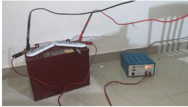
Figure 4.7: Charging Setup of Battery 1.
