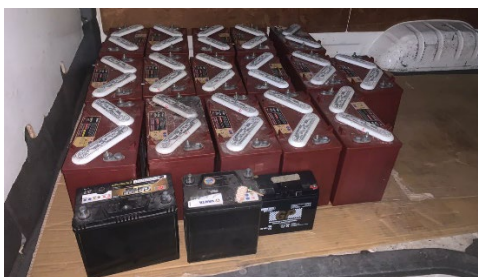
Figure 4.25: The Lead-acid Batteries Loaded into the Cargo Van.
