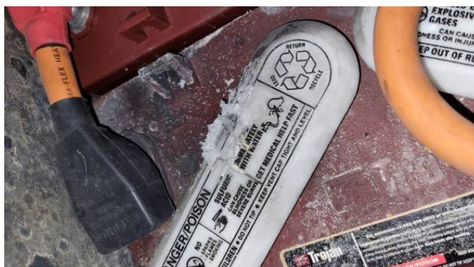
Figure 4.2: White Crystal Solids Deposited on the Vent Cap of Lead-acid Battery.
