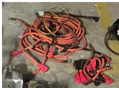
Figure 4.26: The Power Cables Removed from the Electric Vehicle.
