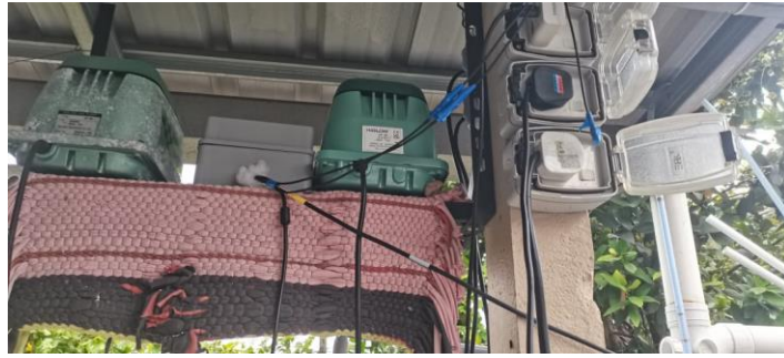
Figure 6.4.2 Junction Box protects the Data Acquisition Module
