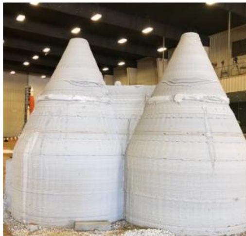
Figure 2: The completed concrete structure produced through 3D printing at the construction site (Muthumanickam et al., n.d.).
