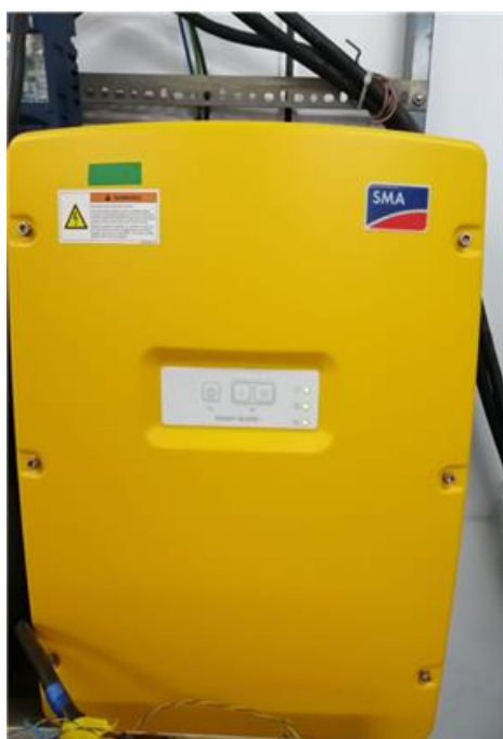
Figure 3.8: Sunny Island Inverter
