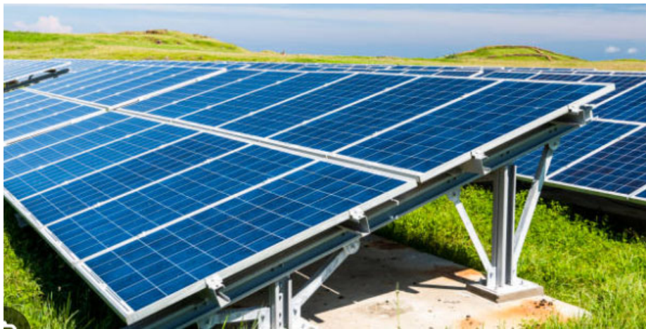
Figure 2.2. Polycrystalline Ground Mounted Installation
