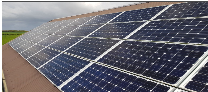
Figure 2.1. Monocrystalline Roof Top Installation
