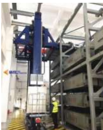
Figure 2.21: A Heavy-Duty Vertical Stacking Battery Swapping Storage (Jasmine Lihua & Danilovic, 2021).
