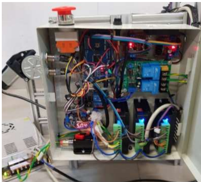
Figure 4.7: All Electronic Components and Wiring in the Control Box Have Been Completed.
