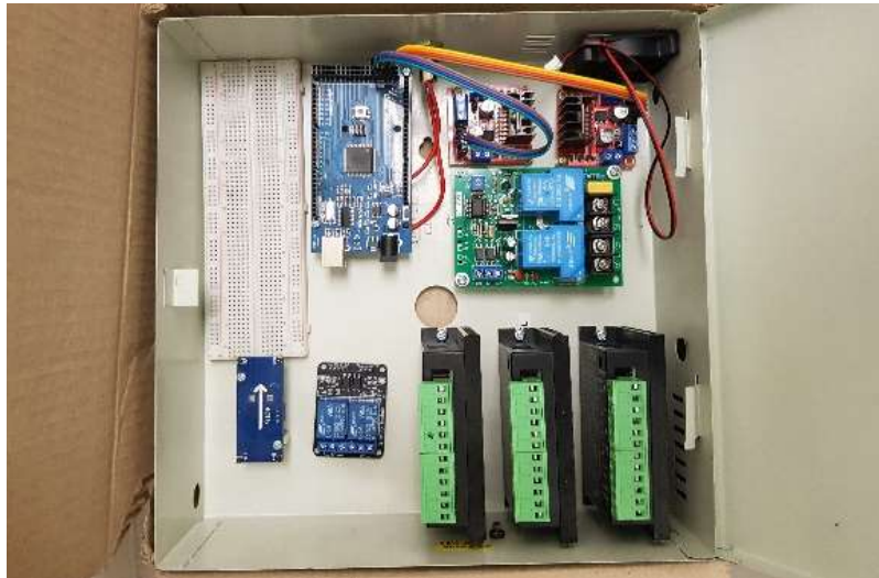
Figure 4.6: The Electronic Components of the Control System Are Arranged Inside the Control Box.
