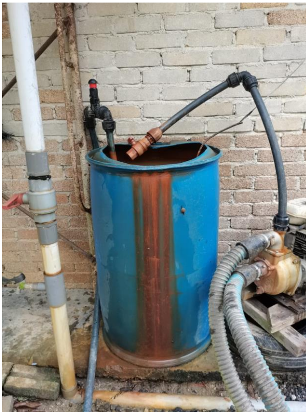
Figure A10: Iron Staining on the Agricultural Appliance
