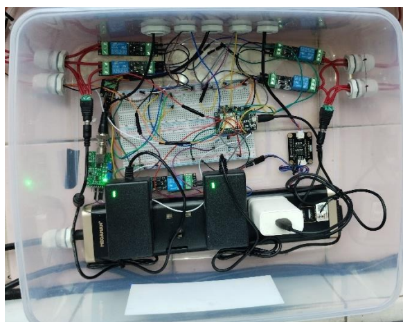
Figure 3.5: Interior of Container
