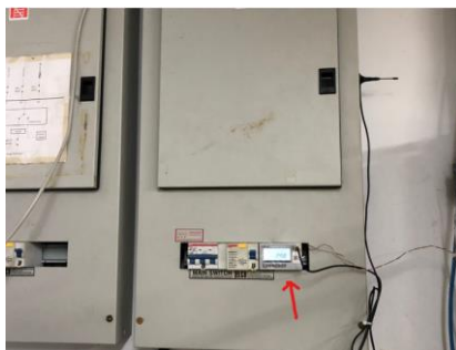
Figure 3.17: Existing installation of the Energy Meter
