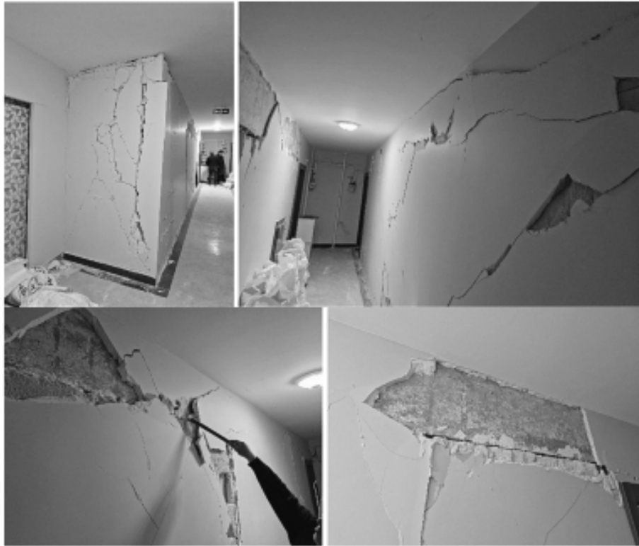
Figure 2. 6: Infill wall damages.
