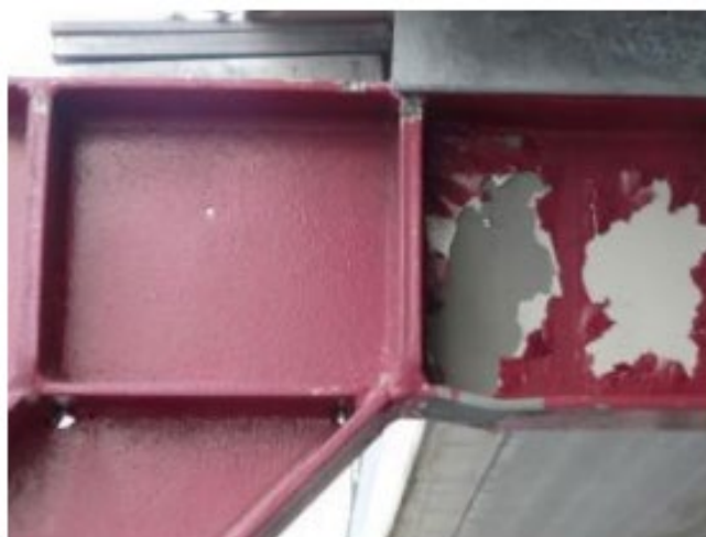
Figure 2. 12: Fractured link at lower level of the EBF.
