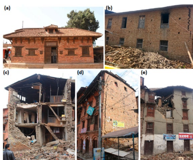
Figure 2. 16: Building types based on nos. of floor: (a) one storey; (b) two storey; (c) three storey; (d) four storey; (e) five storey.
