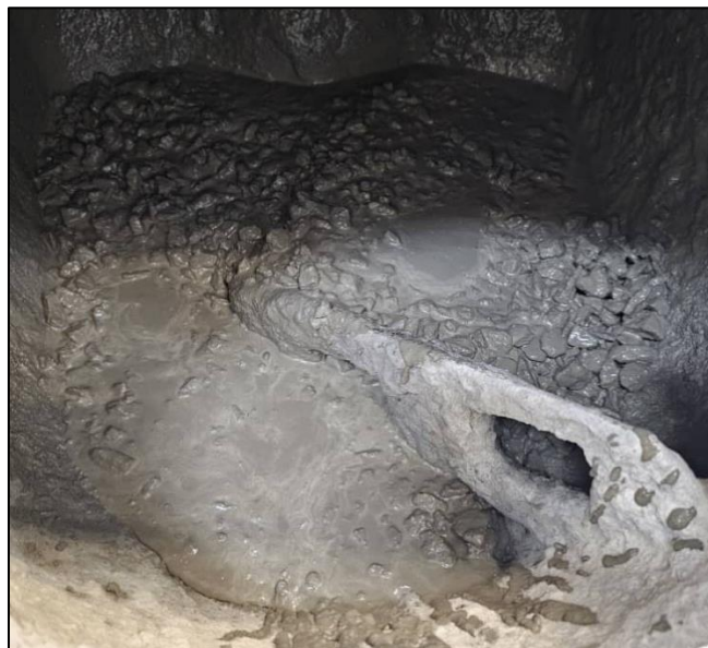
Figure 4.7: Concrete Mix Condition for SP0.6.
