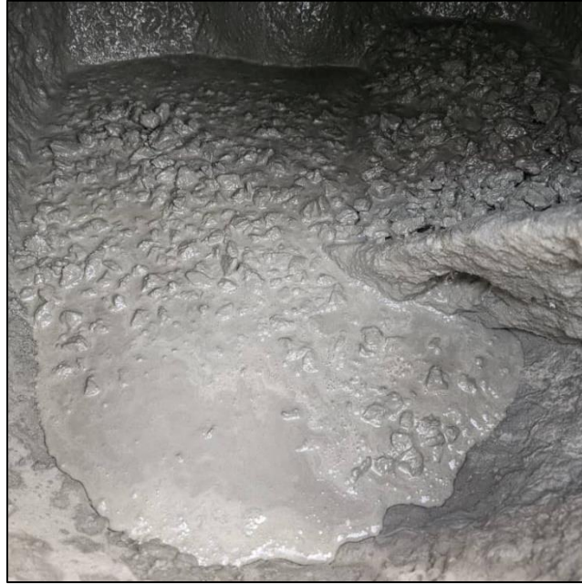
Figure 4.8: Concrete Mix Condition for SP0.7.
