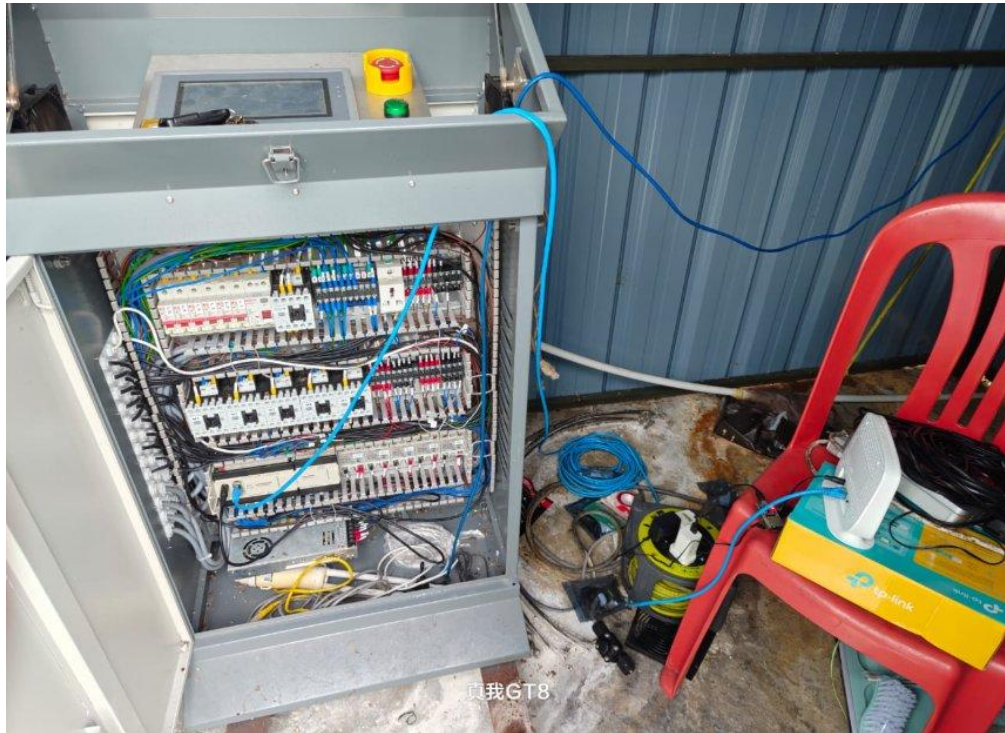
Figure 4.1: Outdoor PLC control panel with AMX-FX3U-M26MR-E PLC and TP-Link MR105 access point at the agricultural park
