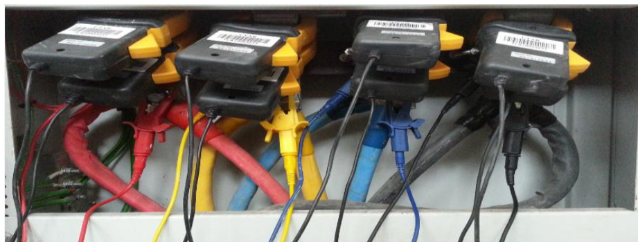
Figure 3.6: Clamping of Current and Voltage Sources from Switchboard
